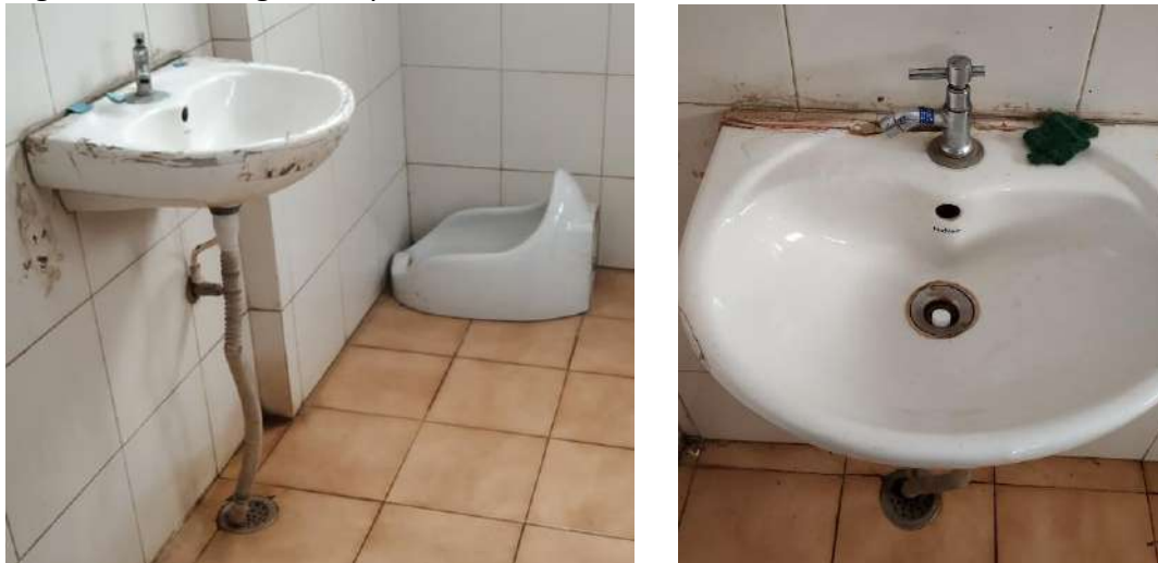
Regular monitoring and repair works are needed
