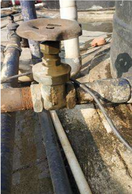
Wastage of water from the valve at roof tank & water cooler
