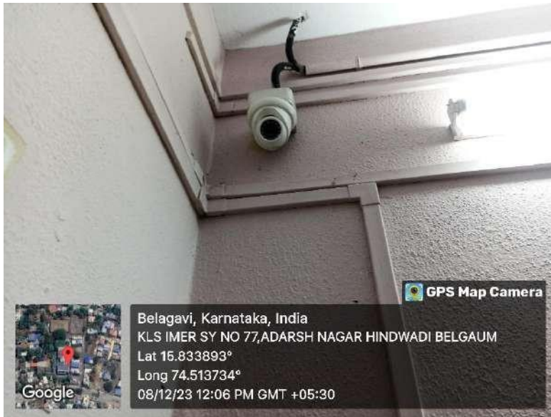
Ladies Hostel Security System
